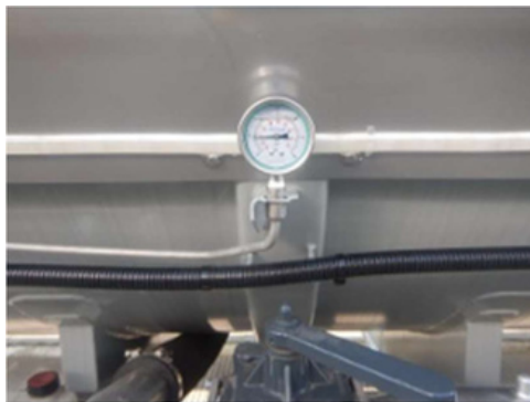
Figure 17: Oil pressure gauge to monitor positive pressure inside tank during discharge cycle
