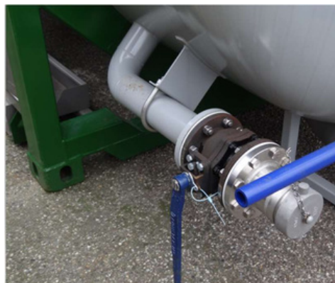
Figure 11: 4" URT product fill line (in closed position)
