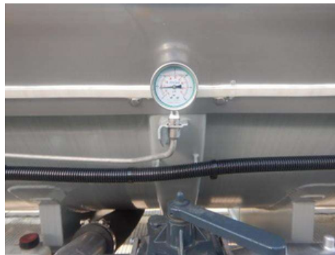
Figure 10: Oil pressure gauge to observe vacuum in tank during fill
