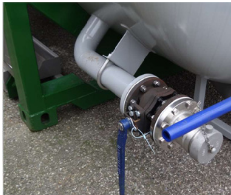
Figure 13: 4" URT product fill line (in closed position)
