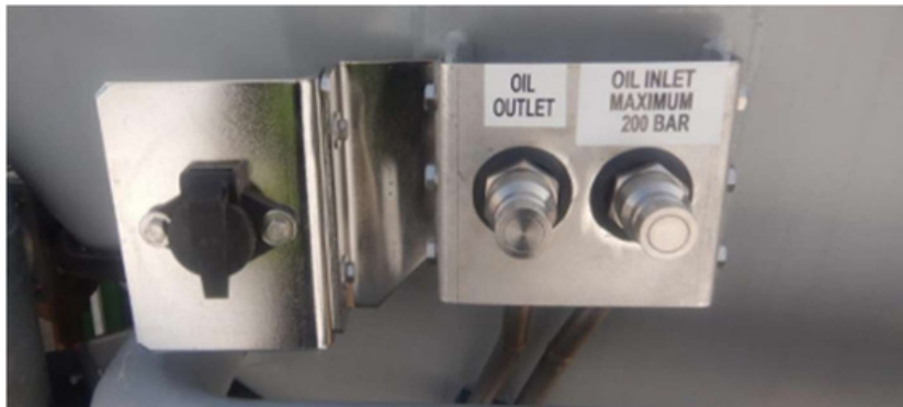
Figure 15: Hydraulic connection points and control switch
